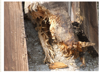
OLD WOOD ROT
